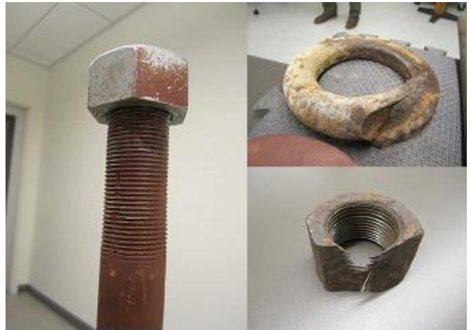
Left: Restored shaft, Upper Right: Piece of broken spring - 6" diameter, Lower Right: Damaged retaining nut
